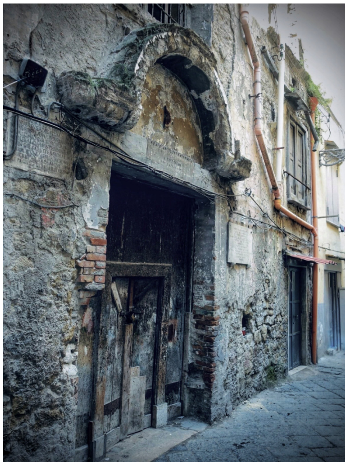
Fig. 6 (A) - Facade of the ancient church of S. Maria a Sicola, today in a complete state of abandonment and decay.
