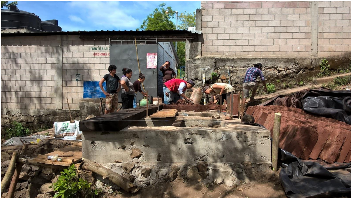
Fig.4 – Laying of the first adobe bricks after the completion of the basement.
