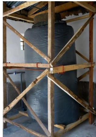
Fig. 3 - Stove fed by biogas and biogas gasometer
