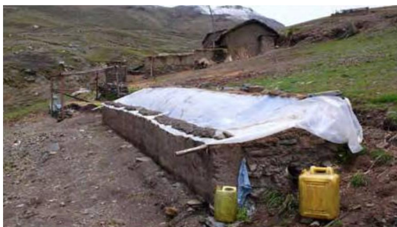
Fig. 1 - Low cost tubular biogas plant
